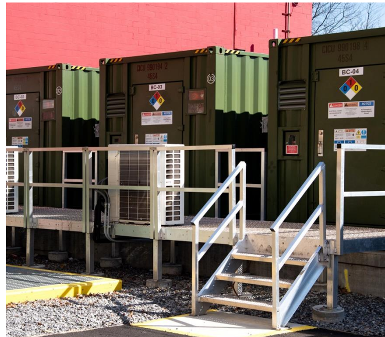
Battery technology from Con Edison's Brooklyn Queens Demand Management Project
