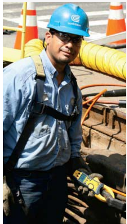
(Top) Robbie Mitchell, meter tester A, at work on the steam system. (Bottom) Jose Montalvo, distribution splicer, takes a load reading on a secondary network cable.
