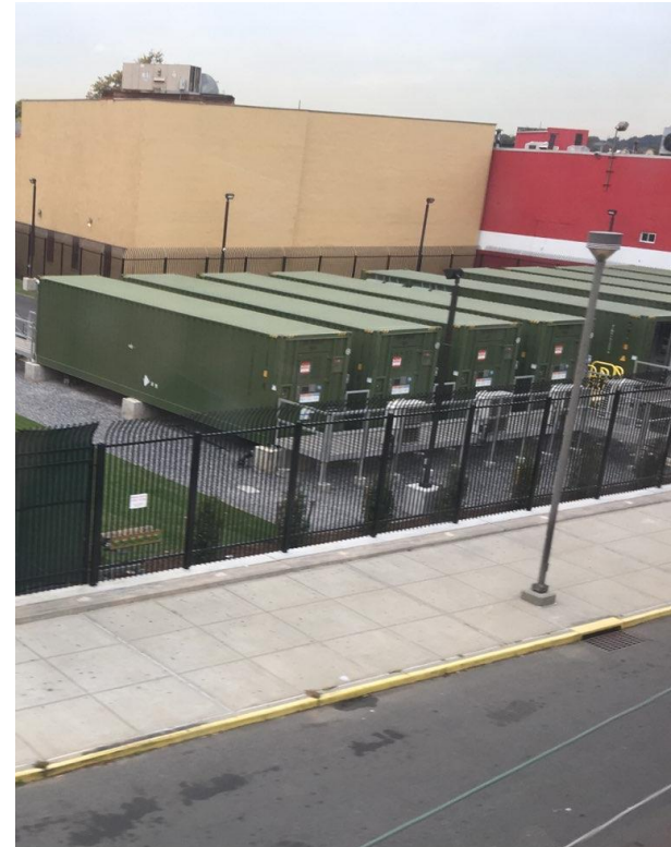
Battery storage is part of the non-wires solutions in the Brooklyn Queens Demand Management ("BQDM") project
