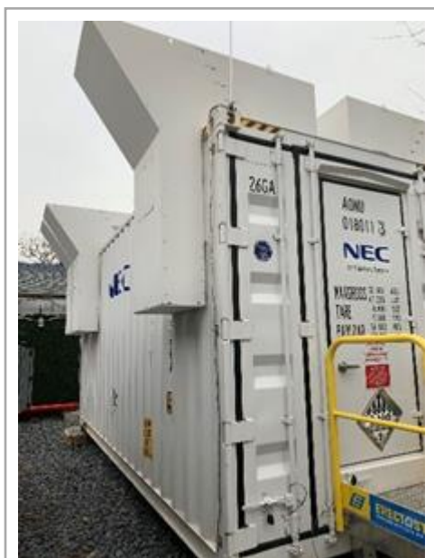
Con Edison has installed a battery to serve customers in a section of Staten Island.
