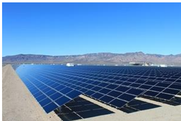
Copper Mountain Solar facility, Nevada
