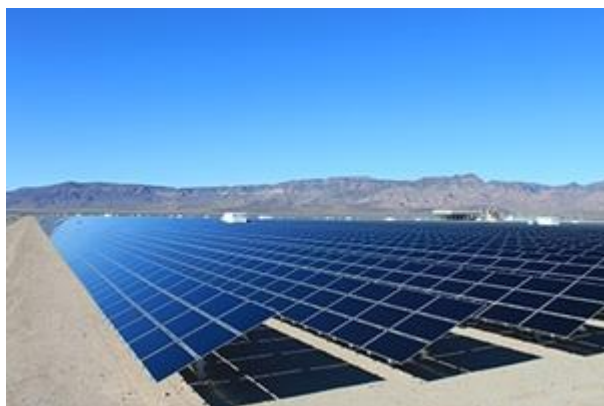
Copper Mountain Solar facility, Nevada
