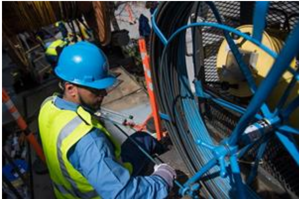
A Con Edison electrical worker at a cable replacement job on the Upper West Side of Manhattan.
